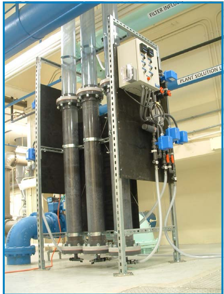
Automated Pilot Filters for Ozone/BAC Pilot
